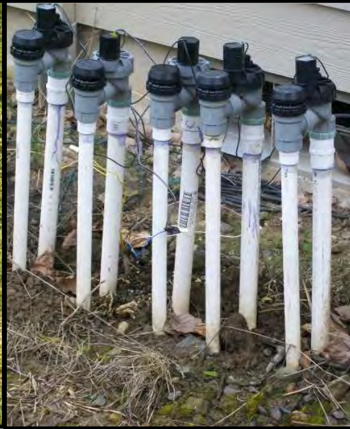
Irrigation controllers w/ Atmospheric Vacuum Breakers (AVBs)
