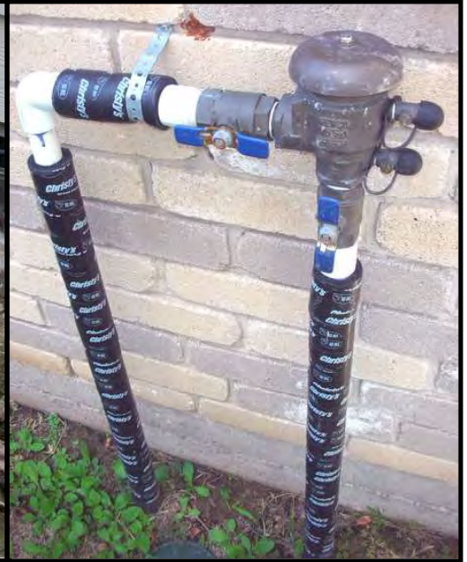
Pressure Vacuum Breaker (PVB)
