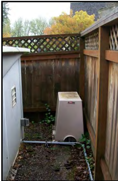
Backflow Assembly in hot box
