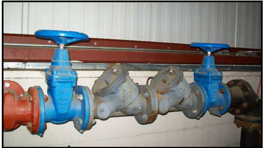
3 inch Reduced Pressure Principle (RP) Backflow Assembly
